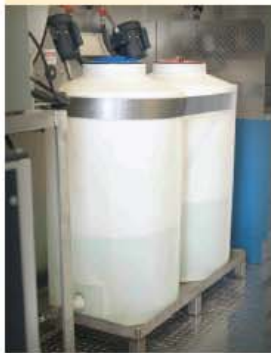
Chemical Mixing Tanks
