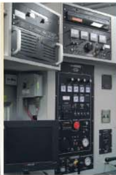
System Control Room
